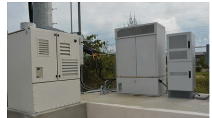
Installations of the Altery Reformer in the Bahamas
